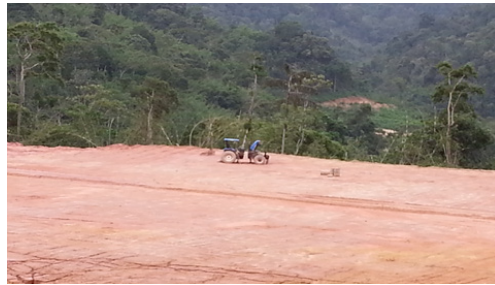
Illegal land clearance at Terisu Post
